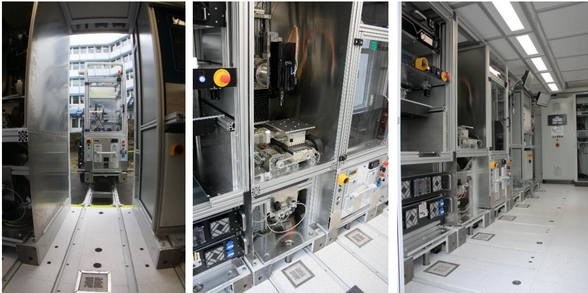
Figure 20: Process module integration (left), installed process modules (middle), view of equipment front and the operator`s corridor (right).
